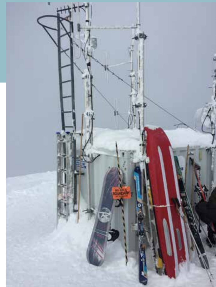
Radio communications tower on the mountain. Photo by John Leonardelli.
